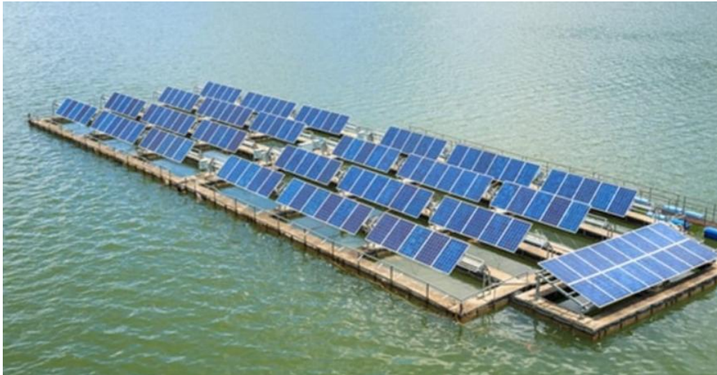
Fig. 5. First Floating Solar PV plant on Chandrika Wewa in the Sabaragamuwa Province, Sri Lanka. Adapted from [23].
