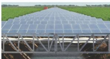
Canal top solar systems
