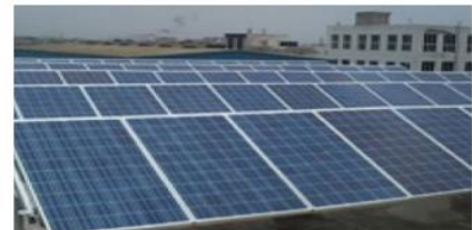
Roof top solar power PV plant
