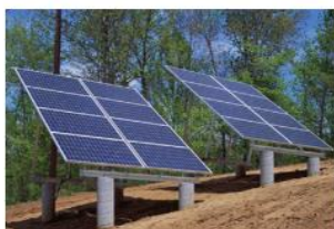
Ground mounted solar PV
