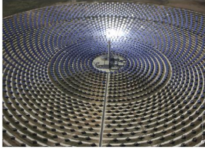
Fig 14. Gema solar power plant, heliostat field, Spain [49]
