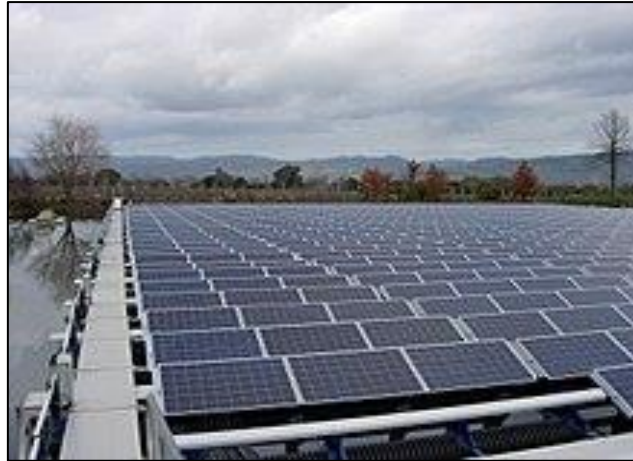
Fig. 13. Floating photovoltaic on an irrigation pond [58]
