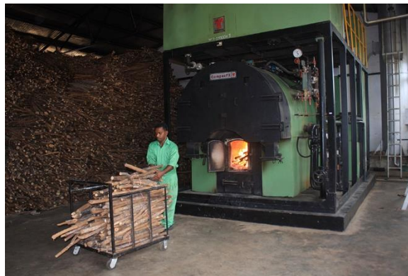
Fig. 3. Biomass (firewood) boiler in Jetwing hotels, Sri Lanka [5]
